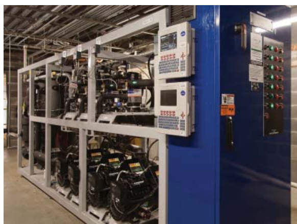
Hillphoenix warm climate CO 2 -based transcritical booster system installation utilizing Emerson components
